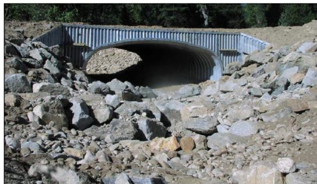
A bottomless arch culvert, shown de-watered for construction, was used to improve fish passage on Hellroaring Creek. This fish passage project was cooperatively funded and implemented by the US Fish and Wildlife Service, Natural Resource Conservation Service, Avista, Idaho Department of Fish and Game, Idaho Office of Species Conservation, and Bonner County Conservation District.
